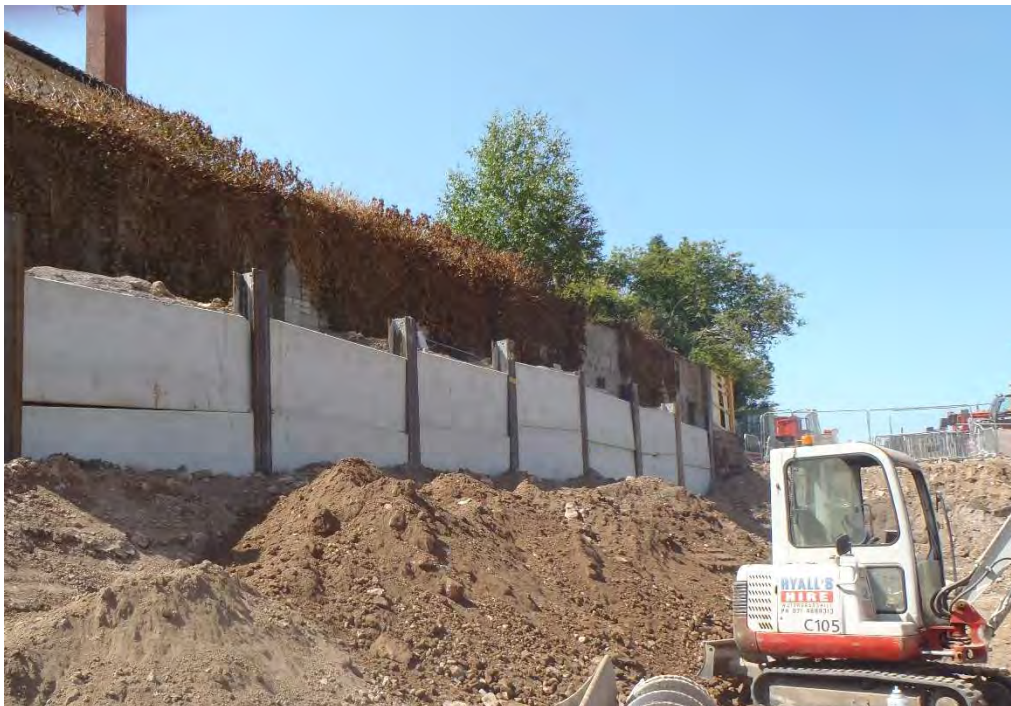
Figure 5-2: Example of a cantilever king post wall with precast concrete infill panels (source AGL)
