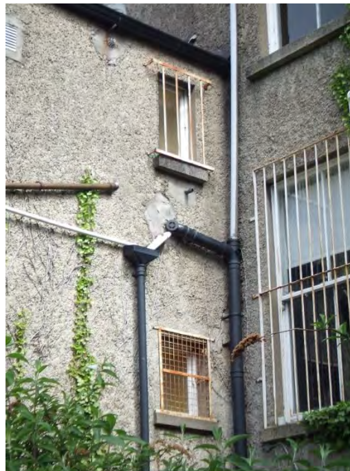
Figure 3-5: Weak point on RHS of Window Reveals
