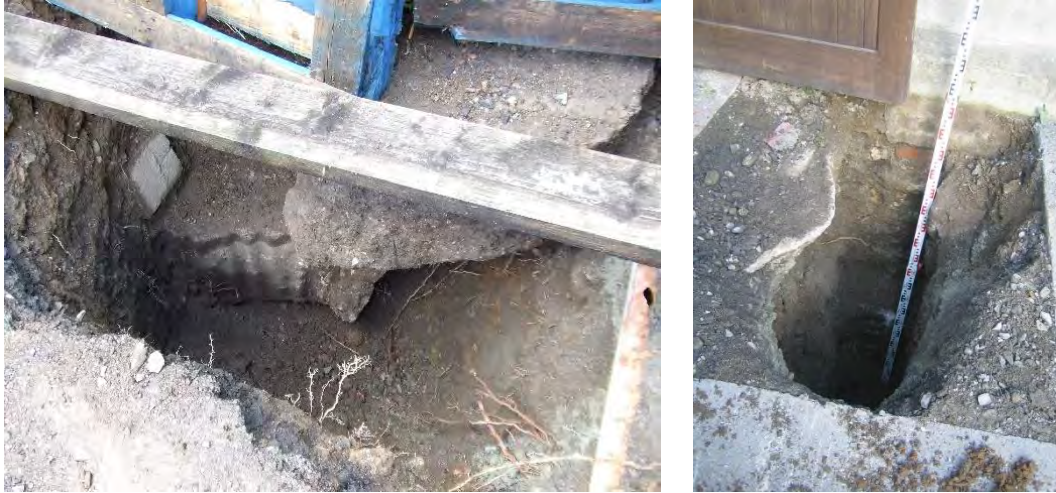
Figure 3-3: Photos of Trial pits at gable wall of return to No.1 Glenville Terrace
