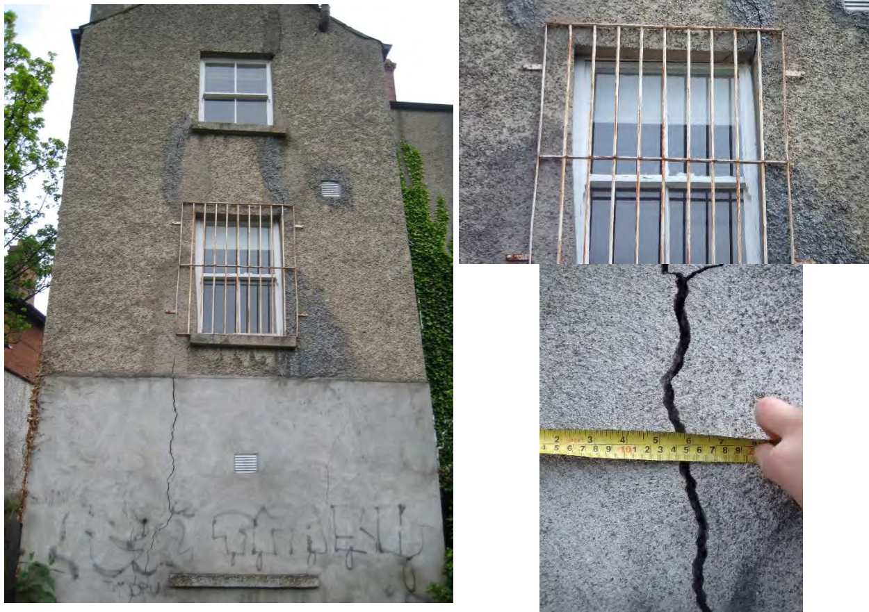
Figure 3-1: No.1 Glenville Terrace Return, Gable wall cracking
